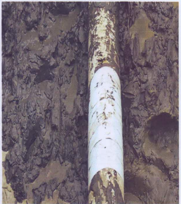
LEAK POINT AFTER REPAIR
